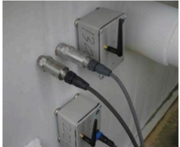
Figure 8 – EPRI’s vibration sensor installed
