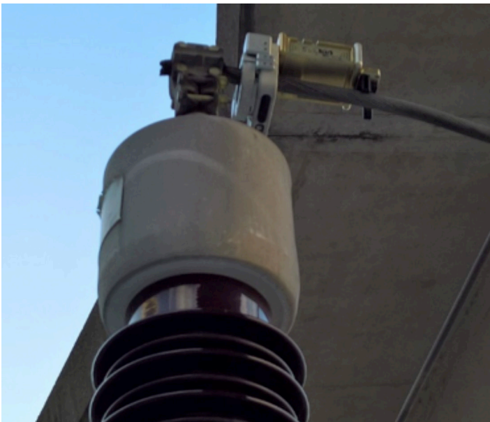
Figure 7 – EPRI’s GIC sensor installed at a transformer high-voltage bushing
